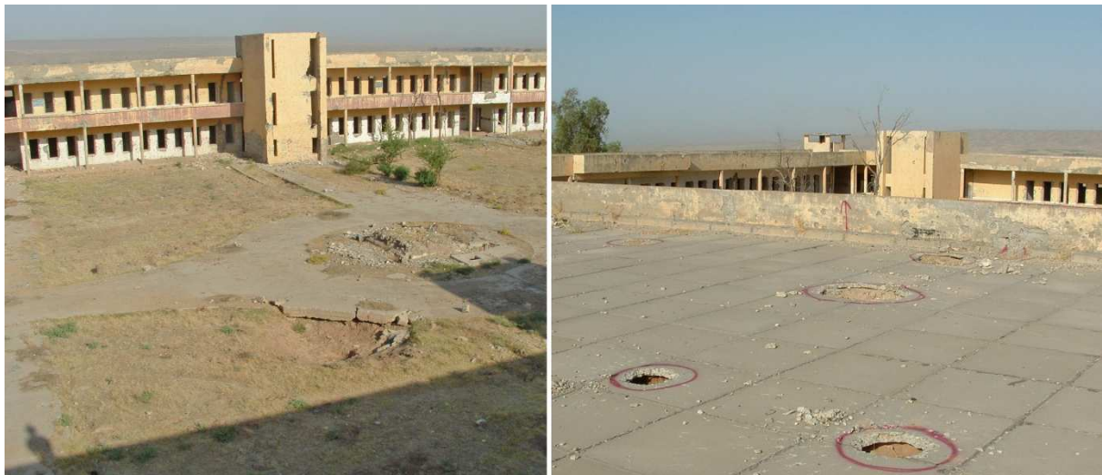
Figure 5: Shows how overhead visibility for a roof inspection can be valuable in a complex urban environment. This example shows evidence of a cluster munition strike. Image credit: Andy Smith.
