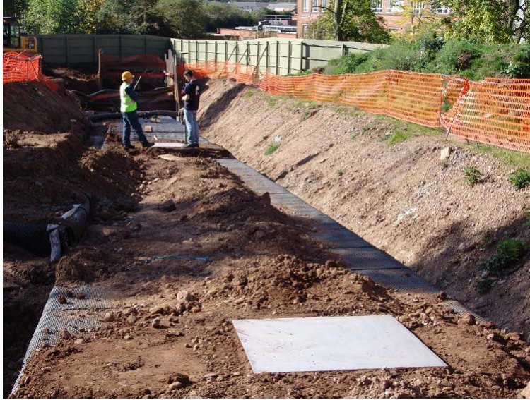
Figure A.1: Photograph of the utility tunnels during their installation. Photograph c/o David Chapman.
