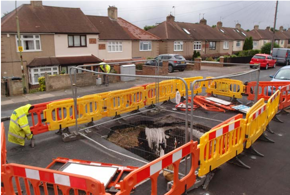
Figure 1.1: A sink-hole causes disruption to a residential road in Dartford.
