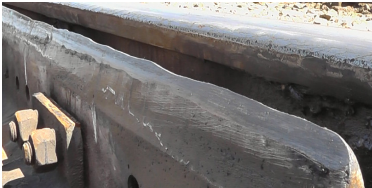
Figure 5-47 Photo of a measured switch (13 PTS, Whitemoor Rail Recycling Centre, photo 1)
