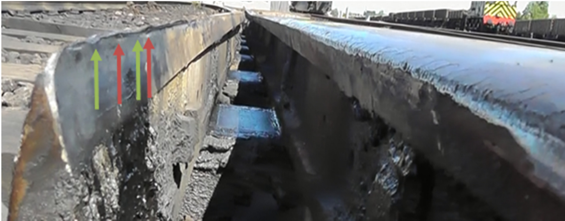
Figure 5-19 A switch that failed Derailment Hazard 1 (photo 1)
