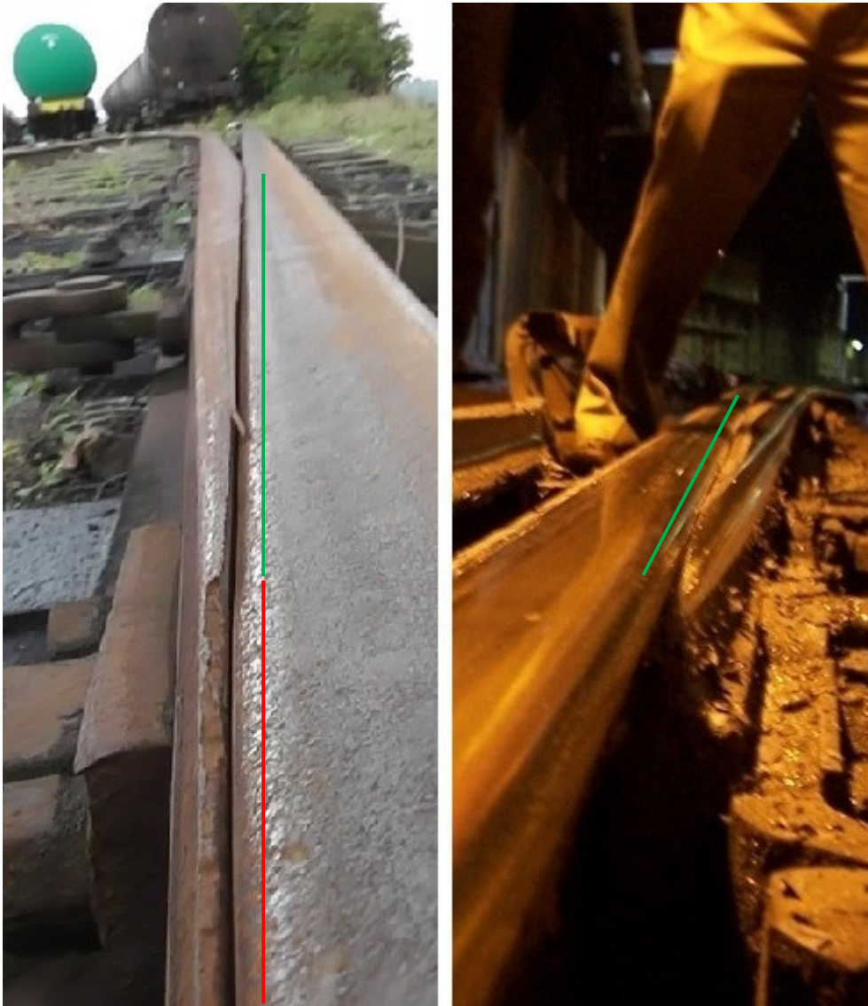
Figure 5-38 Example of damaged switch rail (photos 3 and 4) right: Courtesy and Copyright Joss Apps
