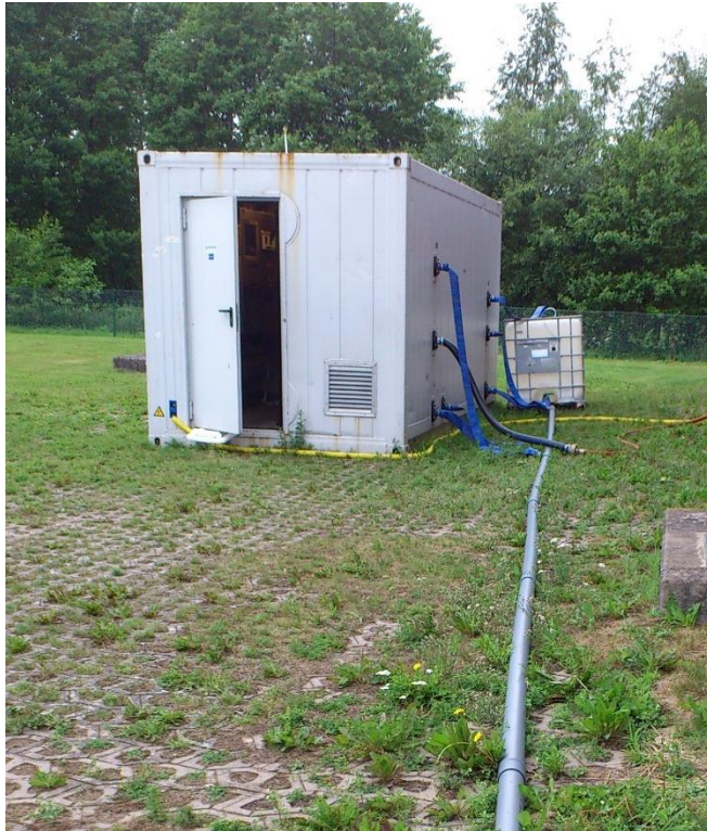
Figure 8 The NF-pilot 80 was located in this container, here placed at the pumping station of Ringsjö WTP.
