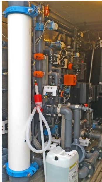
Figure 7 The inside of NF-pilot 80, with the membrane module in the foreground, pumps, valves and tanks can be seen behind it.
