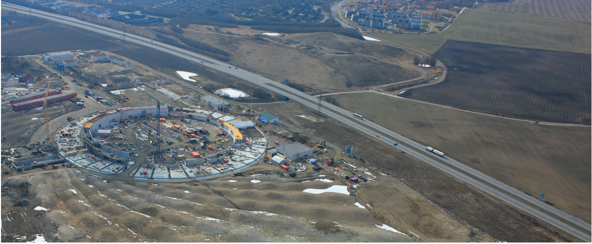
Figure 2.9: An aerial photograph of the MAX IV area and of the E22 motorway nearby in March 2013. Photographer Perry Nordeng.
