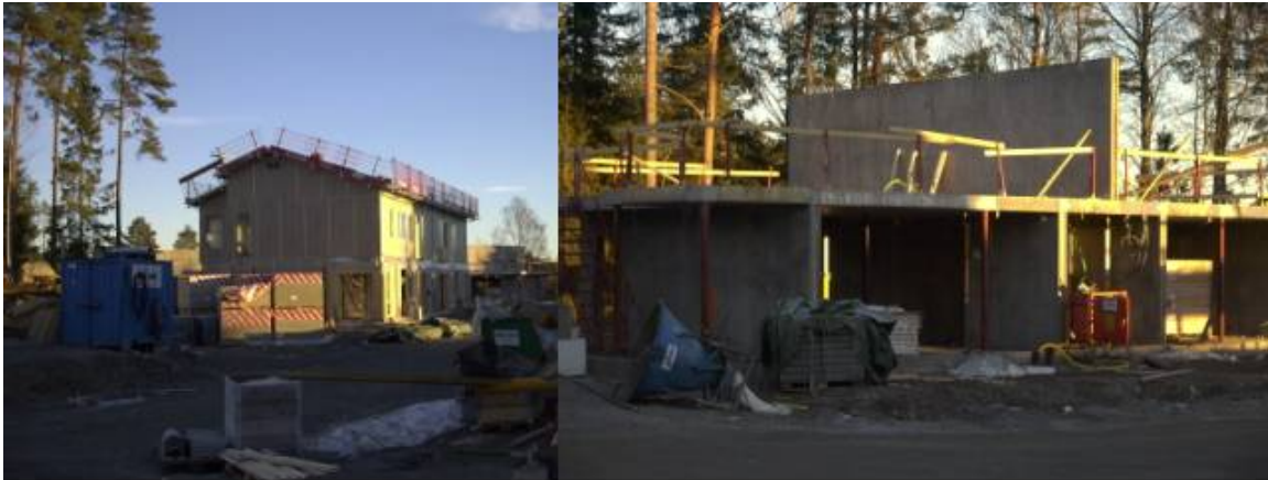
Figure 7.3 Example C during construction. Structural frame to the right. Photos by the author.
