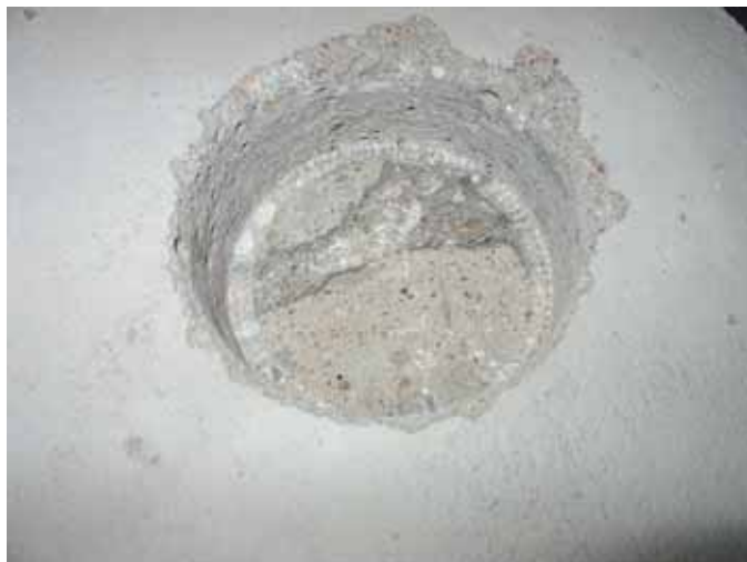
Figure 19. The remaining hole from \varnothing 90 mm core drill, after extracting samples to moisture distribution determination before flooring. Drilling was performed from the top in a homogenous slab from Batch 1. Note the clear breaking zone separating the mortar screed from the concrete material.
