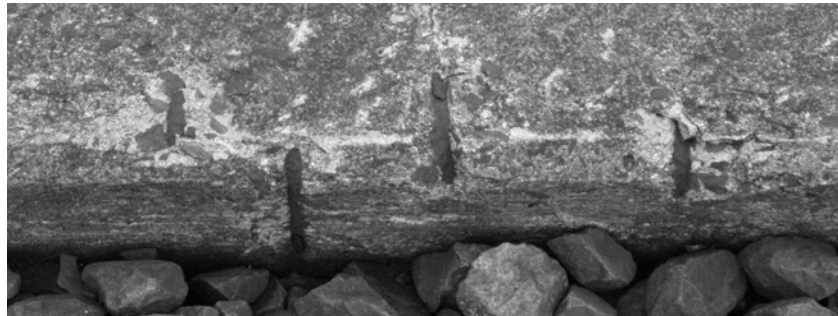
Figure 7.6 Corroding superficial reinforcement at the corner of a girder.
