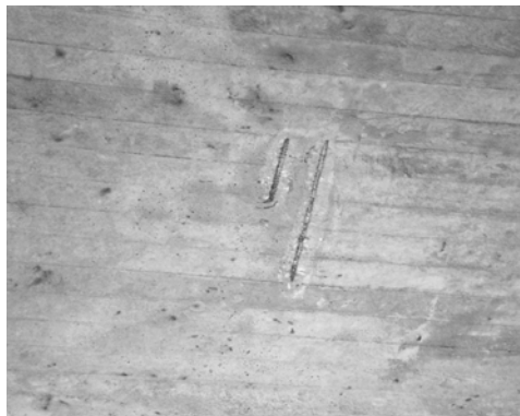
Figure B.3 Large pores and superficial reinforcement that is corroding on the underside of the trough.
