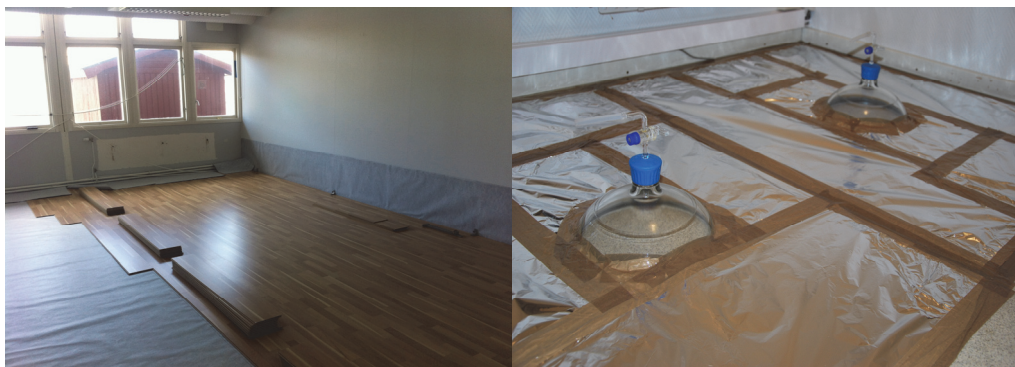
Picture 1. Installation of the cTrap above the source of emissions in a school building (left) and an office room (right, courtesy Jörgen Grantén, Lund, Sweden).
