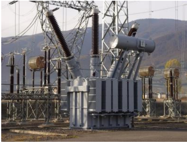
Figure 3. A power transformer in a 63/20 KV substation, West of Mazandaran
