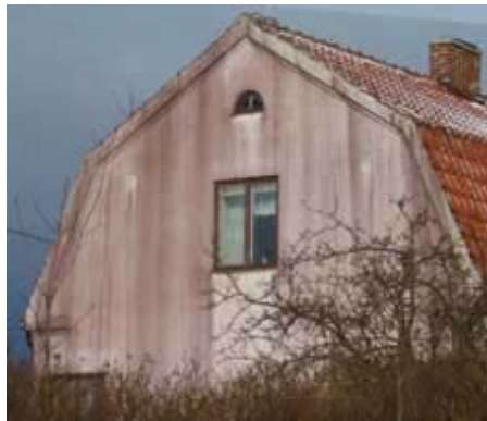
Figure 5.7 Façade of building in Fågeltofta completely covered (except under windows) with Haematococcus pluvialis
