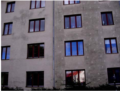
Figure 5.12 Façade of a building in Kristianstad. Left half of the façade with minor discolorations, right half completely discolored and the “white dots” were very distinct
