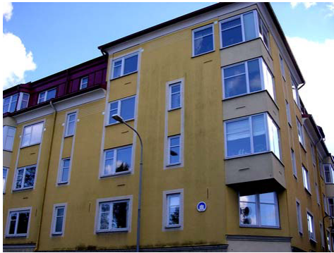
Figure 5.8 Building 1 in Kristianstad with frames of aerated concrete. The yellow façade has discolorations
