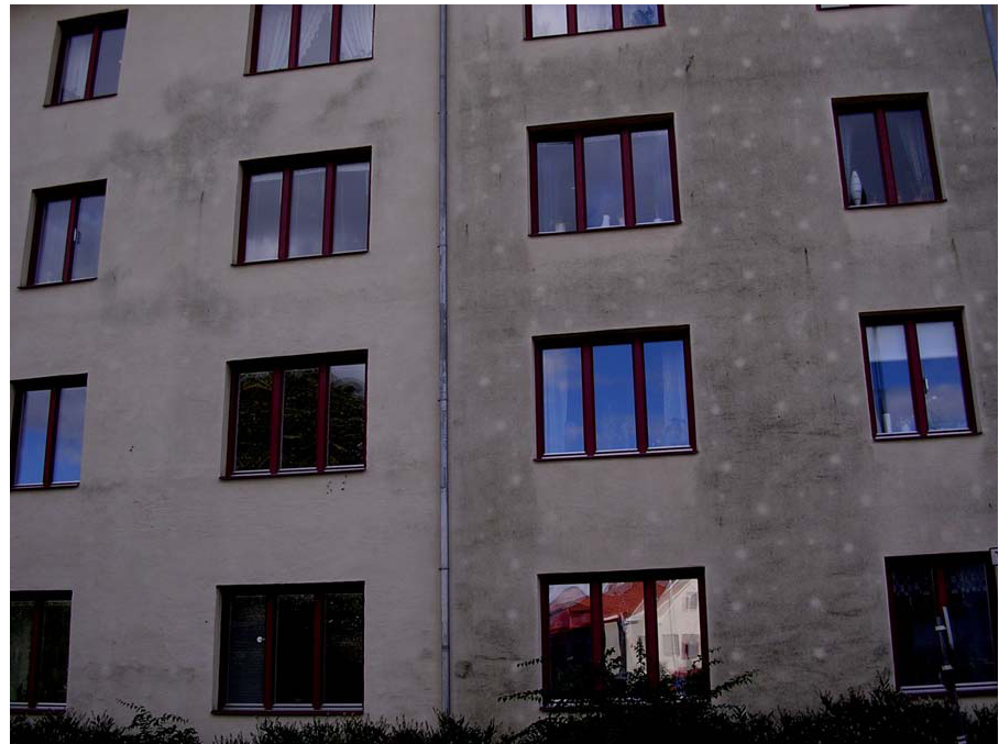
Figure 2 Façade construction with thin rendering on thermal insulation, heavily affected by microbial growth on the right part of the façade. The white dots have no biological growth
