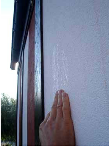
Figure 5.27 The north-facing façade elements were wet as seen with a hand touching the façade the 14 th of September 2006 at 8:30 AM.
