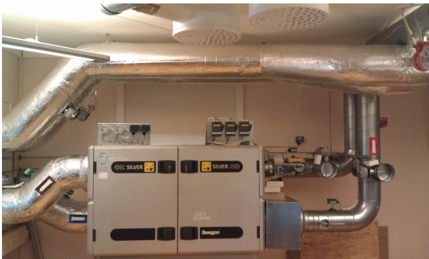
Figure 7.2 The air handling unit.
