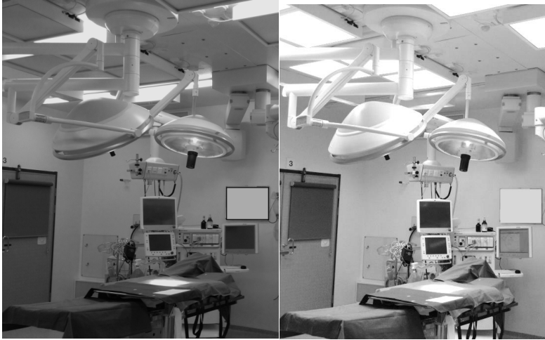
Figure 2. The existing general lighting (left) compared to the test general lighting (right).
