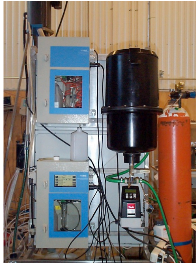
Figure 3.3 Furthest up to the right is the Evita phosphate sensor from Danfoss A/S with its signal converter beneath and to the left is a multi-parameter instrument (ammonia, COD and nitrate) from Awa Instrument.
