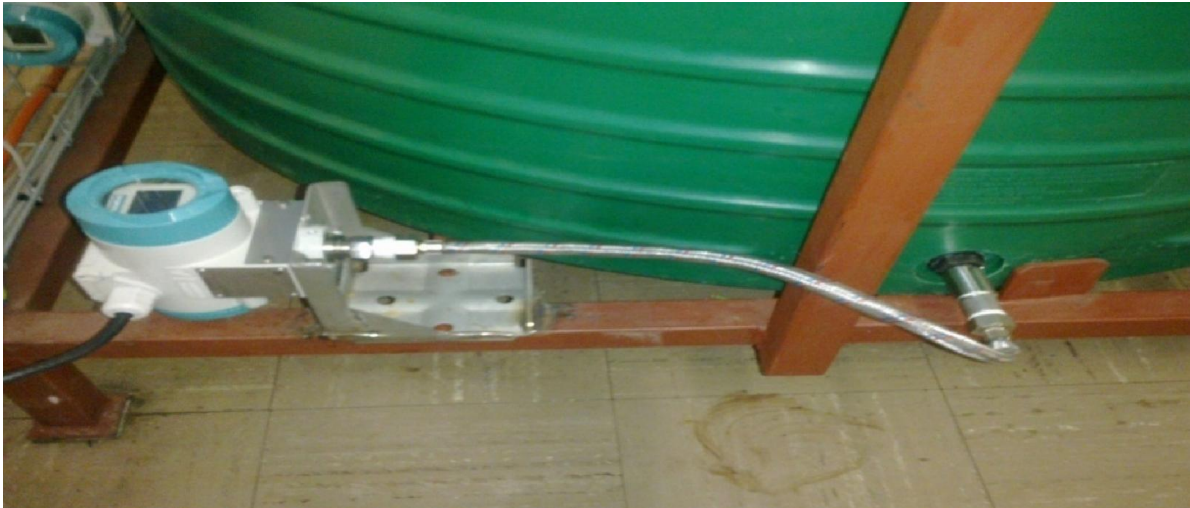
Figure 3.6: The level transmitter is connected as shown in the actual plant.
