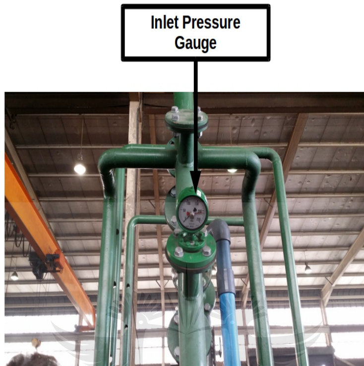
Figure 5.5: Inlet pressure gauge
