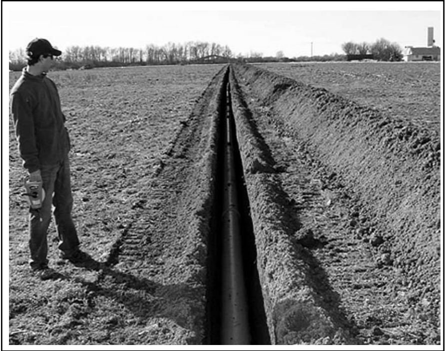
Figure 8. Robin Frazier (NRCS) checks out a pipeline.
