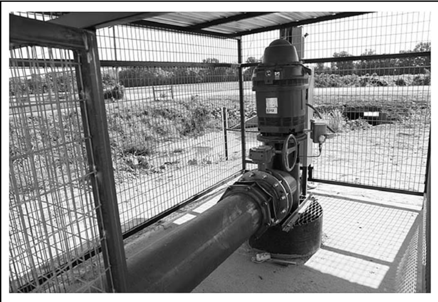
Figure 7. Electric pumping plant.
