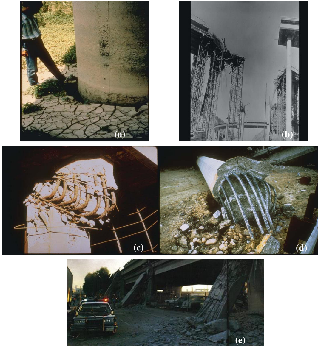
Figure 1- 6: Examples of the substructure damages: (a) Manjil Earthquake (Iran) - Large lateral pier displacement of undamaged concrete bridge, (b) San Fernando earthquake (USA) - collapsed overpasses highway bridges, (c) San Fernando earthquake (USA) – Shear failure due to insufficient transverse reinforcement, (d) San Fernando earthquake (USA) - failure in flexure due to deficient anchorage of longitudinal reinforcement, (e) Loma Prieta earthquake (USA) - collapse of the bridge due to Joint shear failure http://www.ngdc.noaa.gov/hazardimages/picture/list
