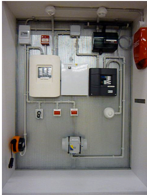
Fig 2. Fire Safety Technical Cabinet.
