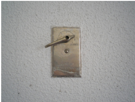
Figure 8. Detail of the manual lever that opens and closes the air-flow vent up to the impulsion grills in each space
