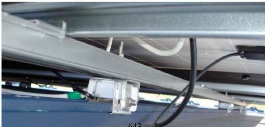
643 Figure 6. Underside of typical Japanese PV array clamp mounting on metal corrugated roof without roof penetration.
