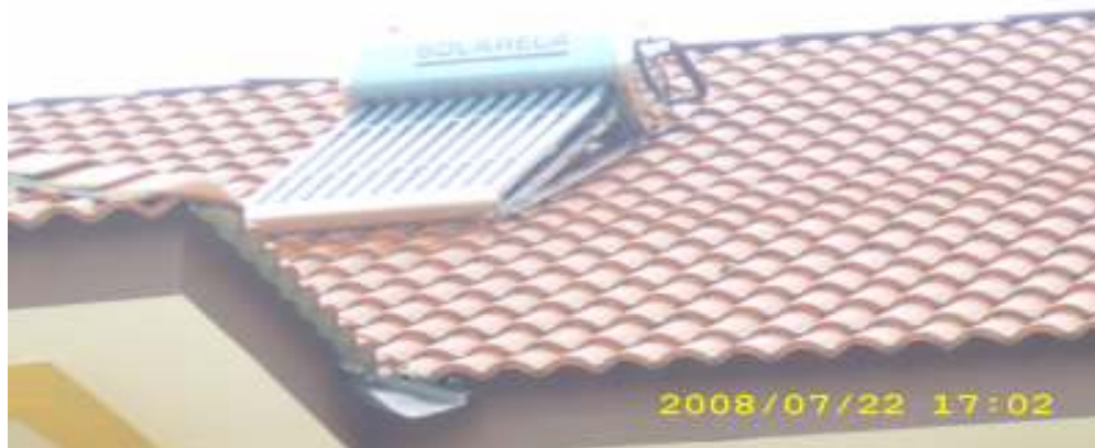
Figure 3.0 : The household in Seberang Perai Selatan, Pulau Pinang which implemented the solar heater system
