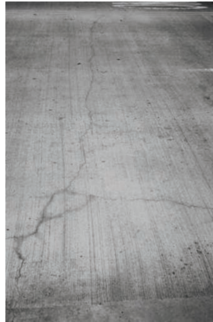
Figure 1.1 Transverse deck crack (Frosch et al., 2010).
