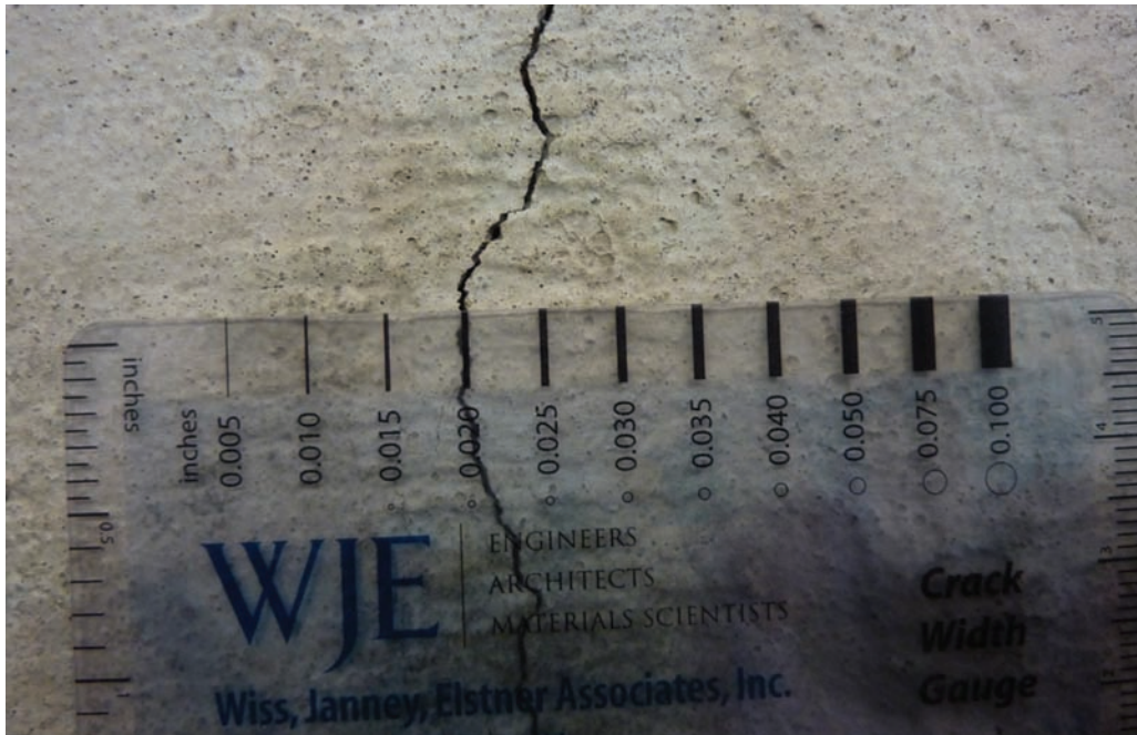
Figure 4.25 Specimen crack measured with crack width gauge.
