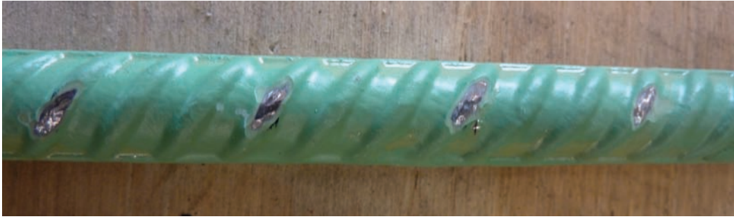
Figure 4.6 1/8 x 1/8 in. damage areas on transverse bar.
