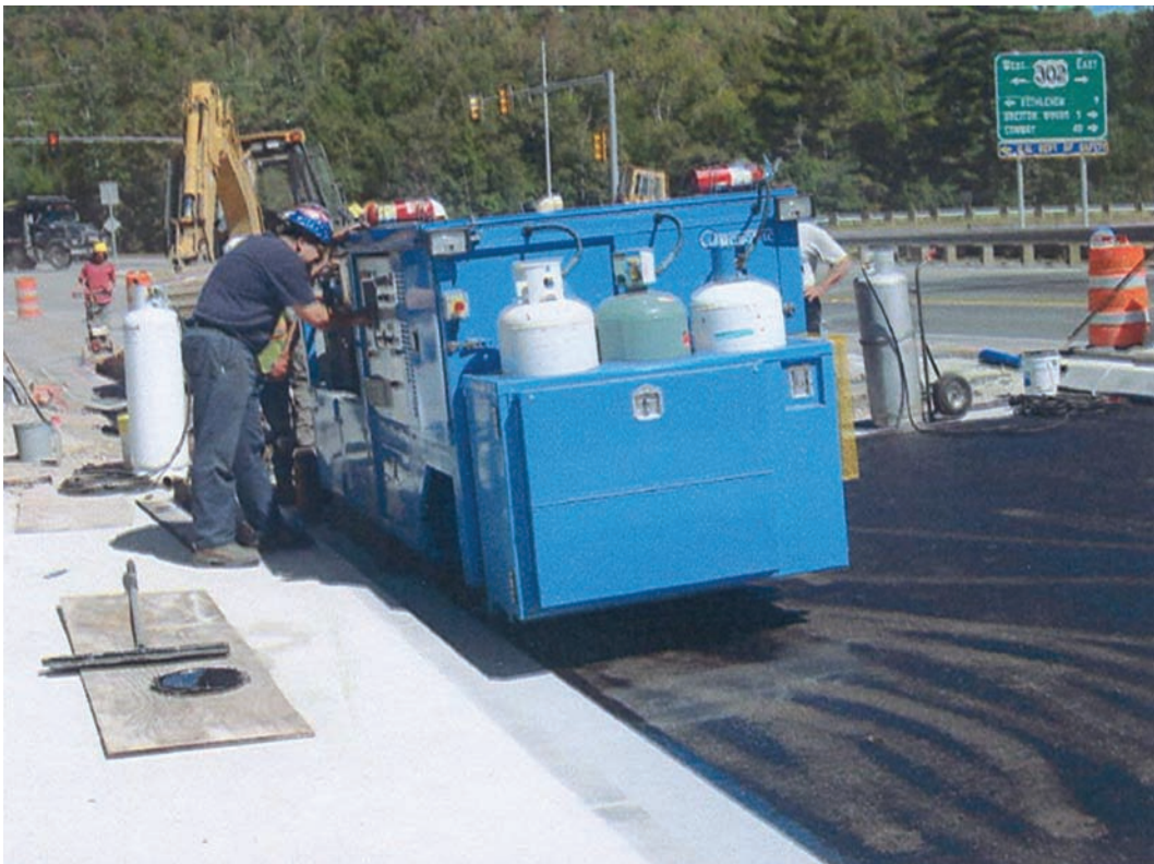
Figure A.13 Membrane application machine.
