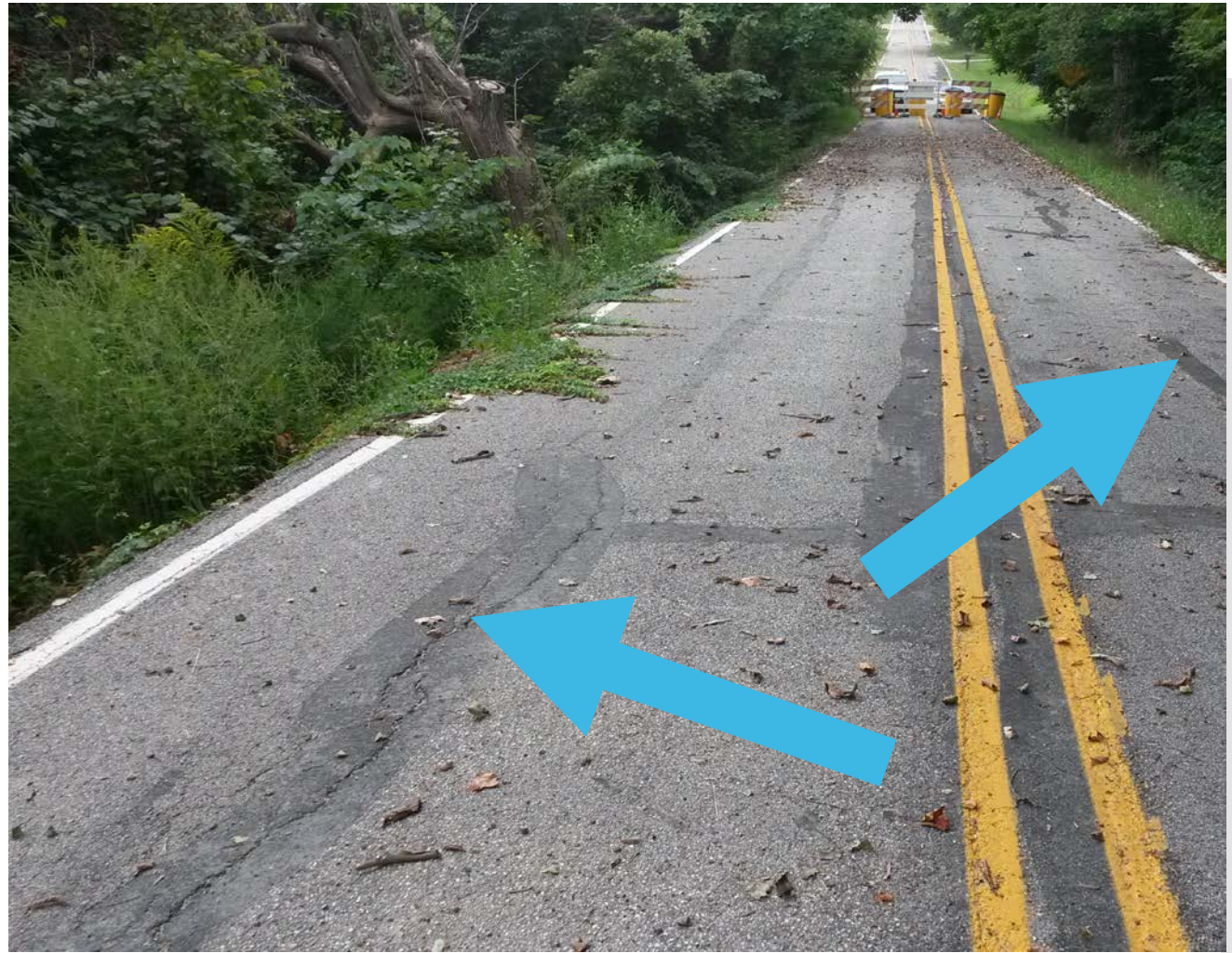
Picture looking South – Crack along EOPs
