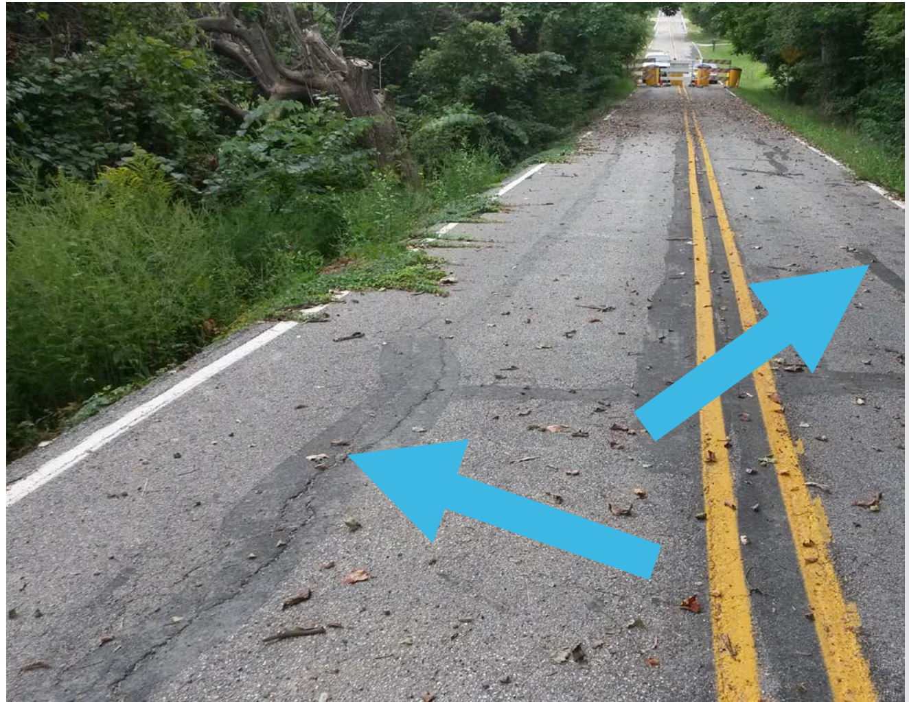
Picture looking South – Crack along EOPs
