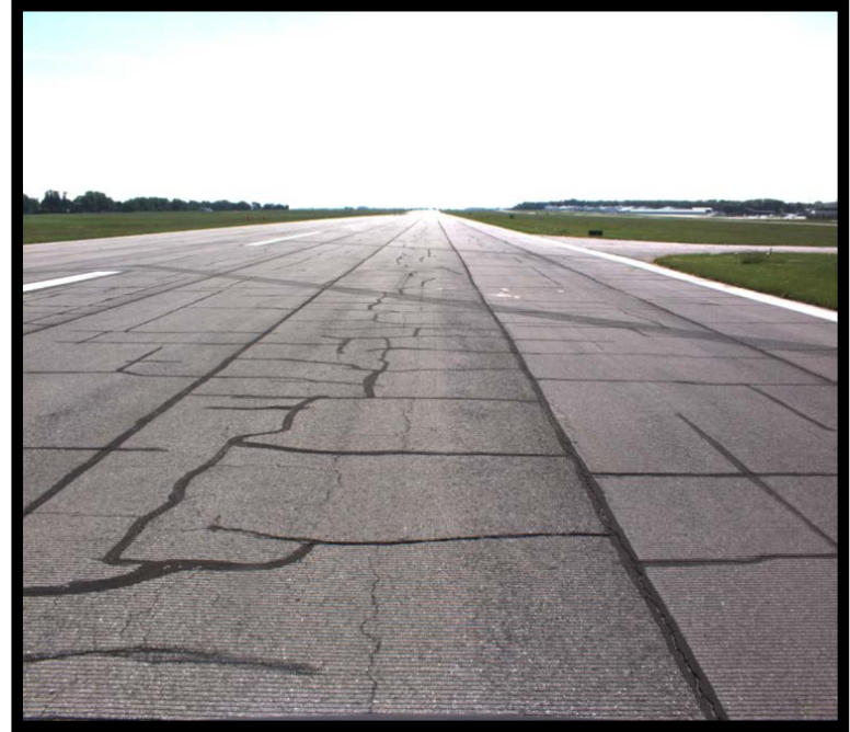
Failing Pavement: Runway 9-27
