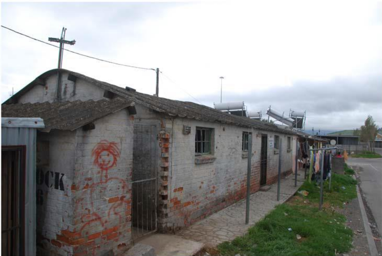
Figure 6. Hostel site before restoration commenced, March 2009. Experienced building contractor, Jerry Rogers, conservation architect William Martinson and industrial archaeologist David Worth visited hostel 33 and gave advice on how to proceed with the restoration of the decaying fabric of the low-spec building. Copyright, William Martinson.
