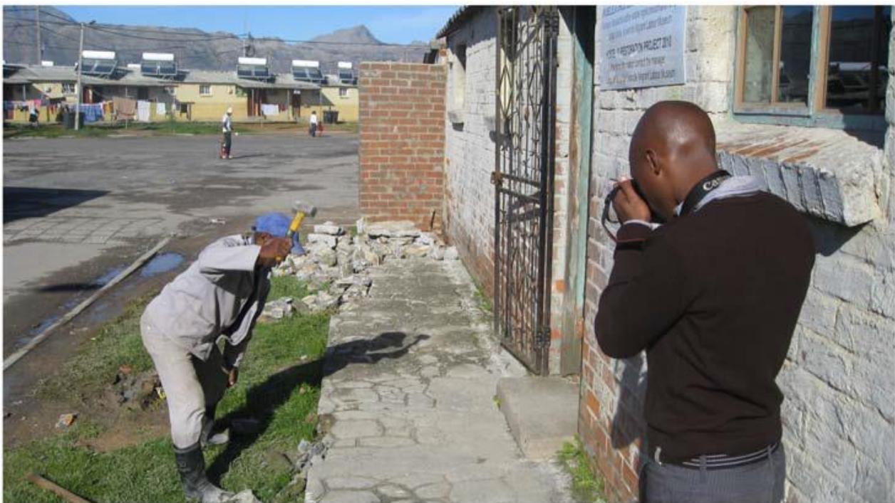
Figure 7. Hostel 33 additions dismantled. Museum staff member Phumzi Nzuzo documents the removal of the concrete apron, June 2010. Copyright, Noëleen Murray.
