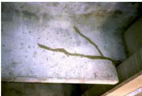
(e) Typical crack at dapped end member
