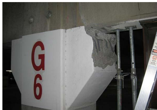
(f) Spalled reinforced concrete corbel
