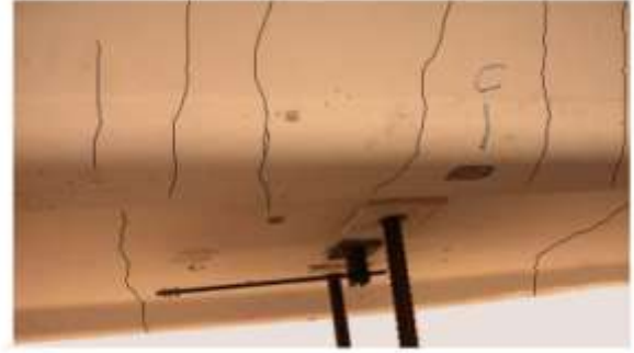
Figure 2: HPSFRC prestressed roof element: cross-section (a) and crack pattern (b) [2].
