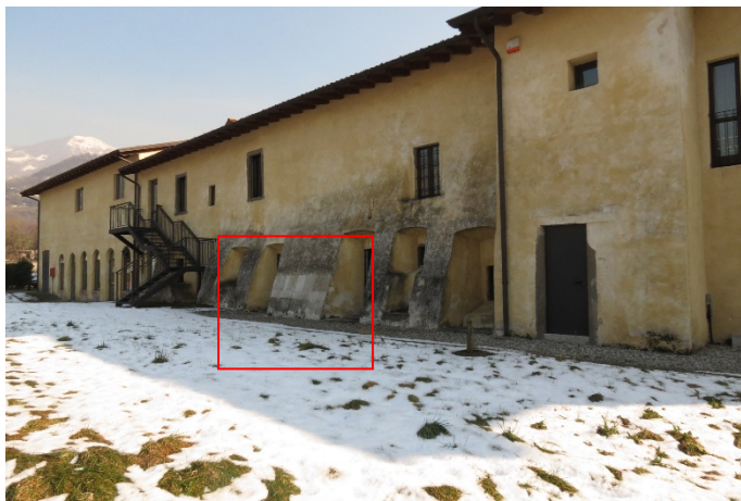
Figure 1 Lavello Convent, Calolziocorte: Northern side. The square frames the areas of application of the biocides under test
