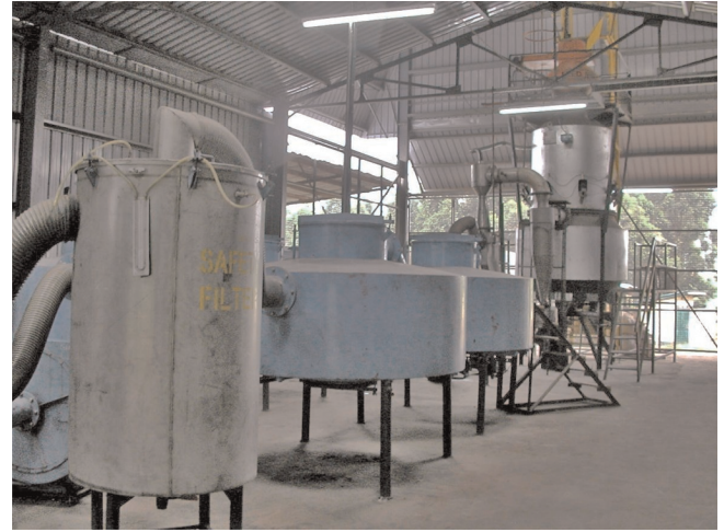
Figure 3. The filter line and WBG 400 gasifier at Muzizi Tea Estate
