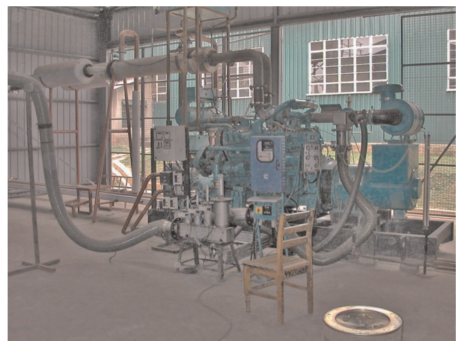
Figure 4. 250 kW producer-gas engine with heat exchangers (upper left corner at exhaust pipe, heat exchanger at cooling cycle covered by control units) at Muzizi Tea Estate
