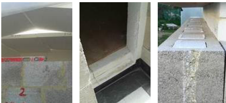
Fig. 3. Test cell construction in progress (a) ceiling level, left; (b) floor level and surrounding walls, centre; (c) capping of cavities of the hollow concrete block at top level, right.
