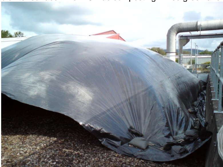
The inflated sheet covering the biofilter surface; odour samples were collected of the escaping air.
