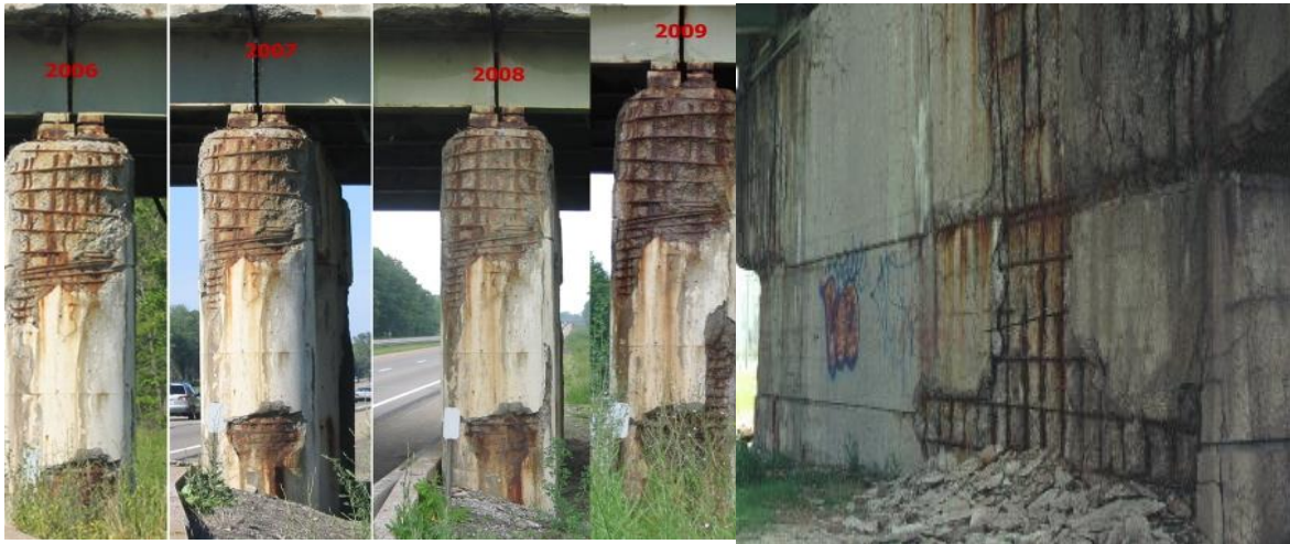
Figure 6.1: Example of problematic concrete structure where the deterioration of rebars and concrete cover spalling occurred [5]
