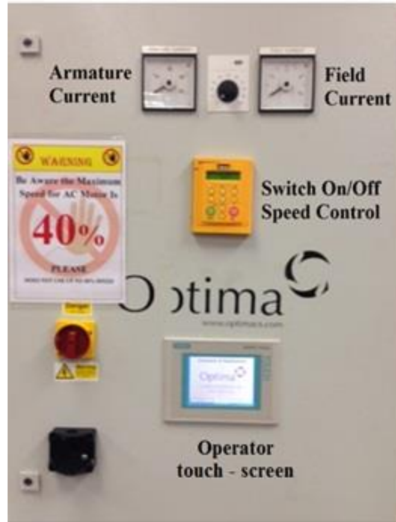
Figure 5.15 The test rig control panel
