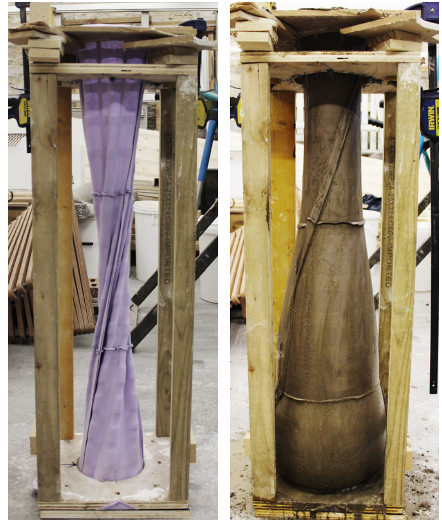
Figure 2. Twisted column. Fabric formwork and wooden structure, before and after the concrete casting of a twisted column. Prior to the casting, the fabric has to firmly stretched. The inside of the fabric formwork contains a 3D printed patterning, used for influencing both the surface texture of the concrete and the stretching behaviour of the fabric. Photo: Cristina Nan.
