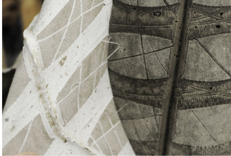
Figure 9. Twisted Column. Removal of the fabric formwork with 3D printed patterning. Photo: Cristina Nan.
