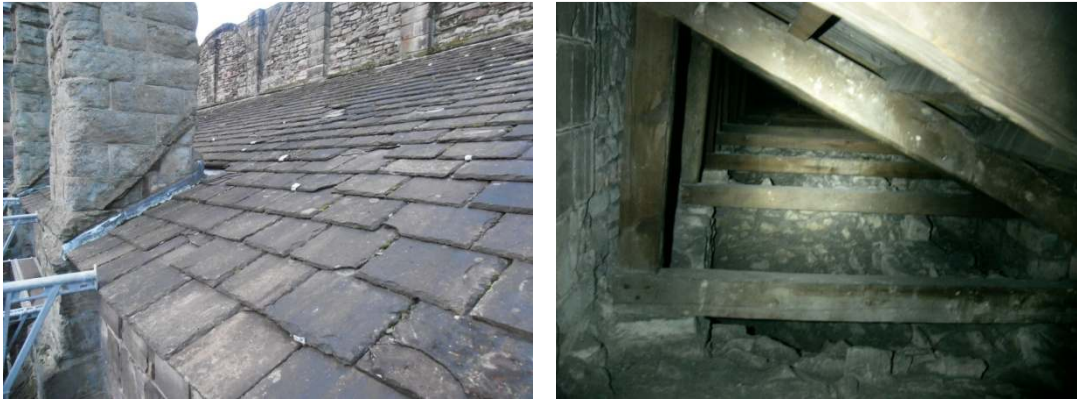
Figure 6. Aisle roof: Covering with stone tiles, similar to what probably used to cover the nave, and internal view of the intrados space (taken in Summer 2013).
