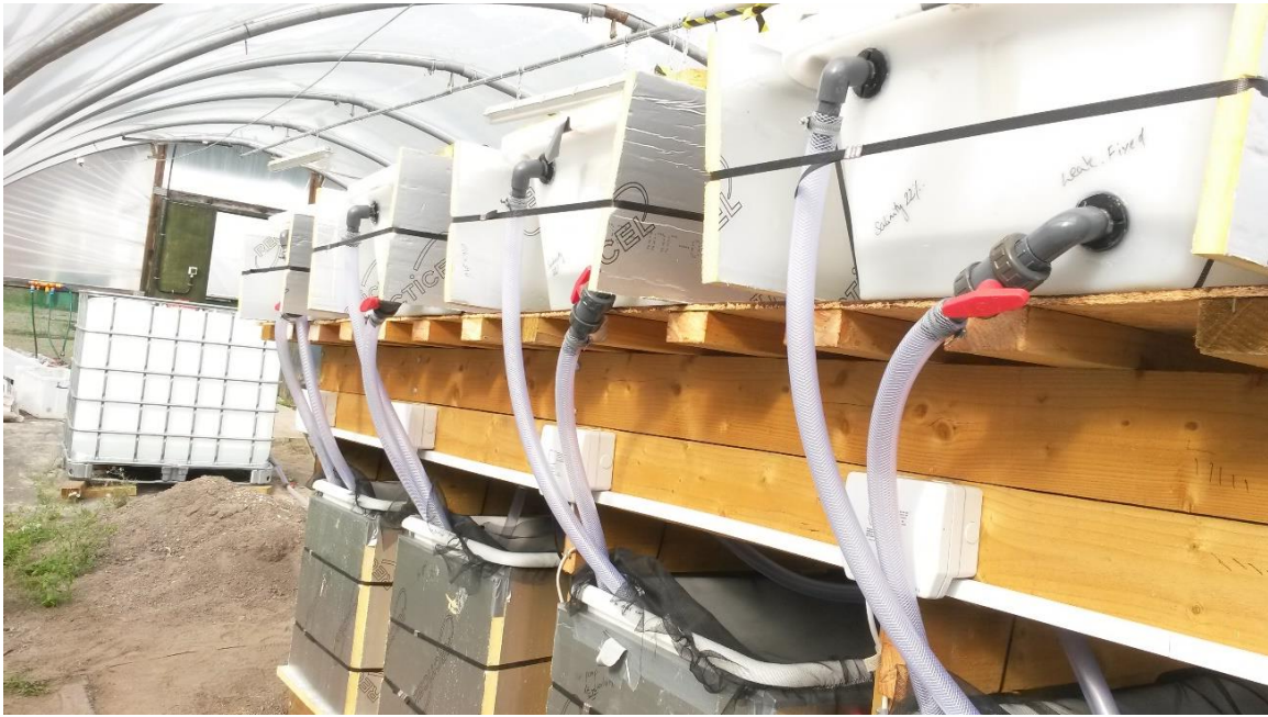
Figure 4.7. Upper and lower tanks showing tubing connections and insulation
