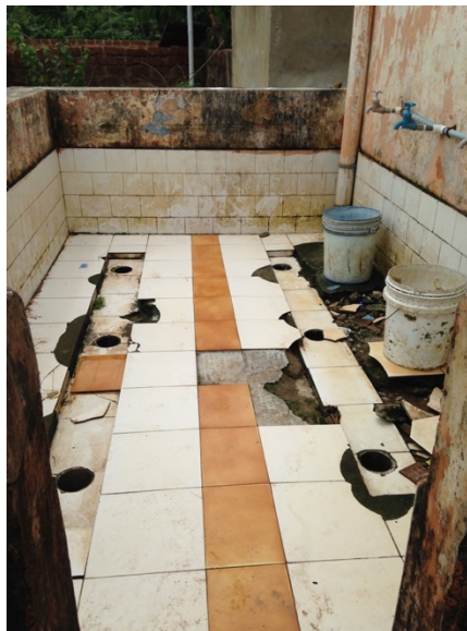
Figure 4.3: Unused and non-functional child-specific latrines at a communal latrine in a slum
