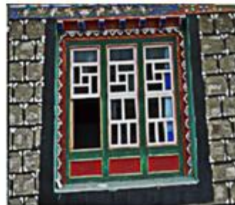
Small areas of windows and doors.
