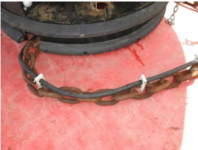
Figure 2: Buoy-to-Hub cable inside hydraulic hose clamped to mooring chain
