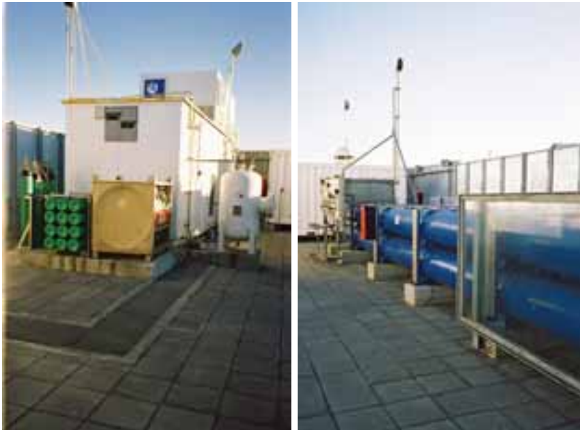
Figure 2.20 Interior views of the hydrogen filling station in Reykjavik: on the left the electrolyser and compressor modules and on the right the main storage tanks and associated pipework
