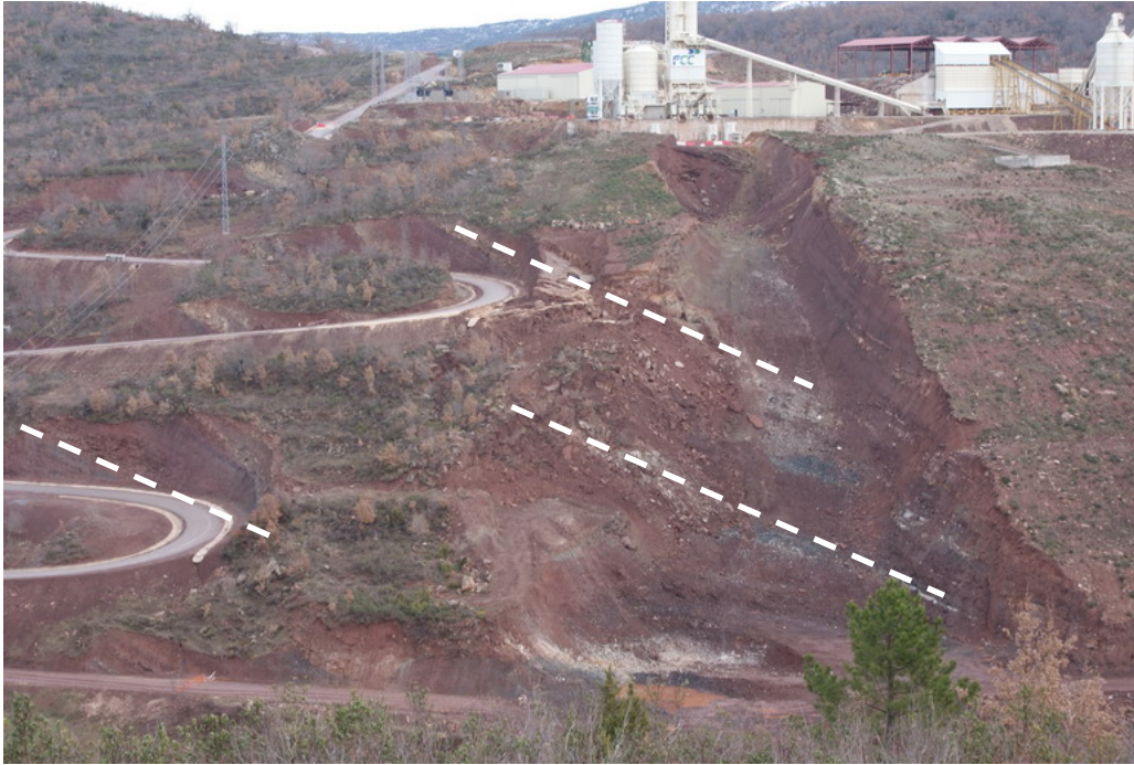
Figure 19: Planar failure in Castrovido claystone controlled by sedimentation planes
