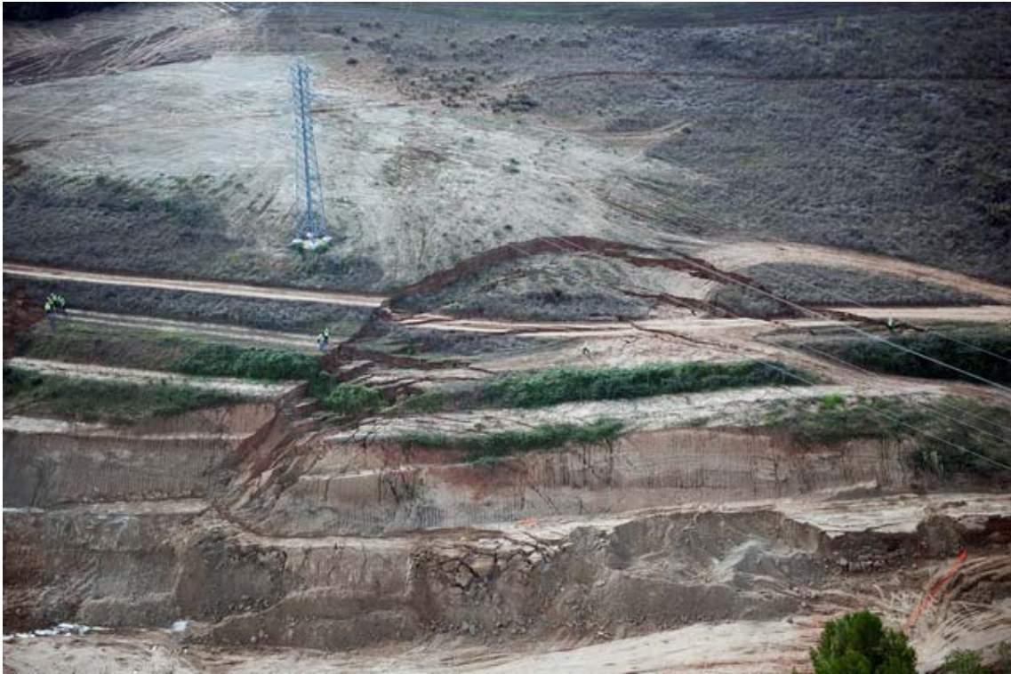
Figure 4: Sabadell slope failure
