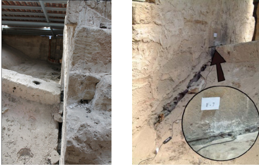
Figure 14. The crack between the third arch and the fourth vault (left) and a zoom to the static monitoring sensor (right).
