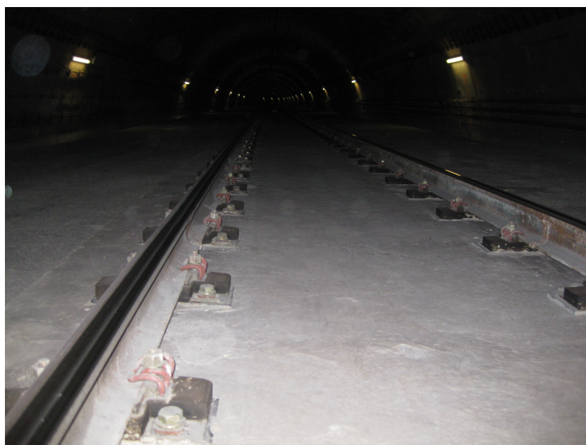
FIG. 6.1: Direct Fixation Fasteners (DFF) used in Line 9 of Barcelona Underground System.
