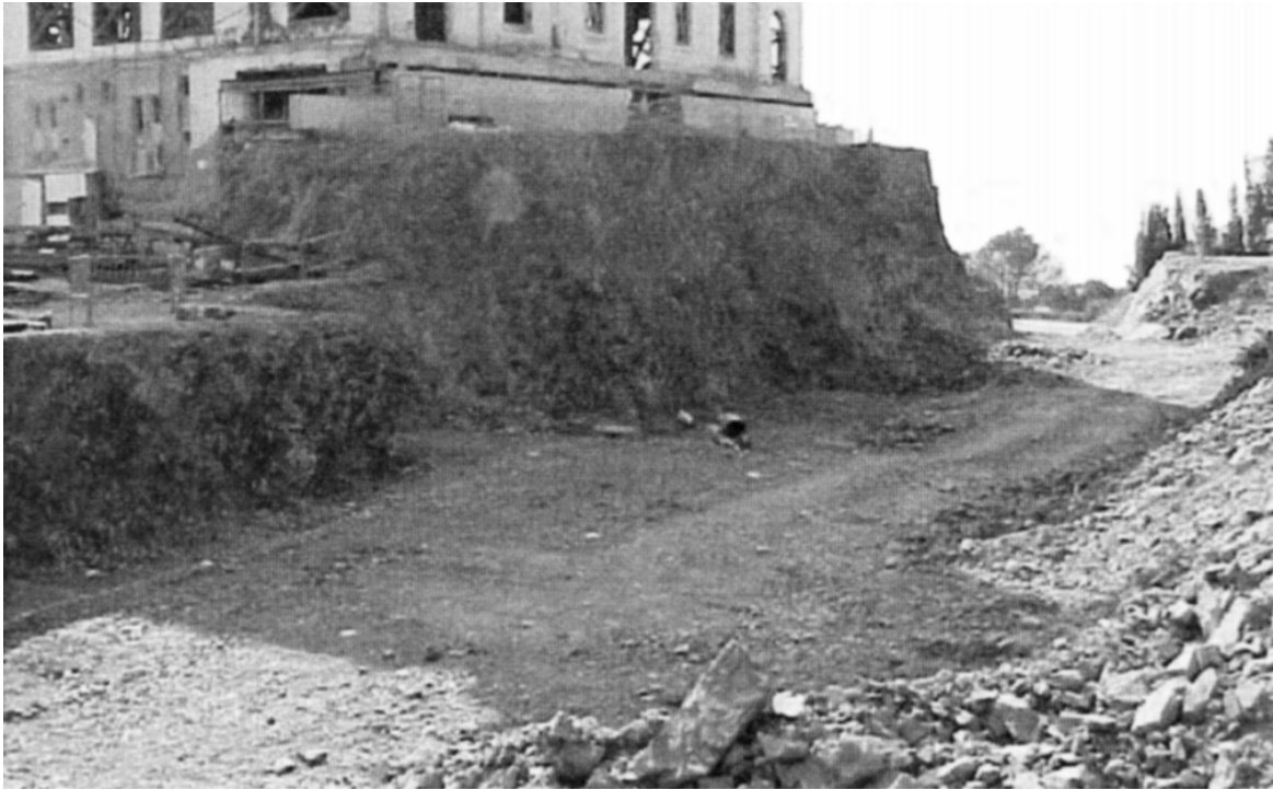
Figure 6. View of the excavation zone before the wall was initiated. The location of the failure is on the right of the image.
