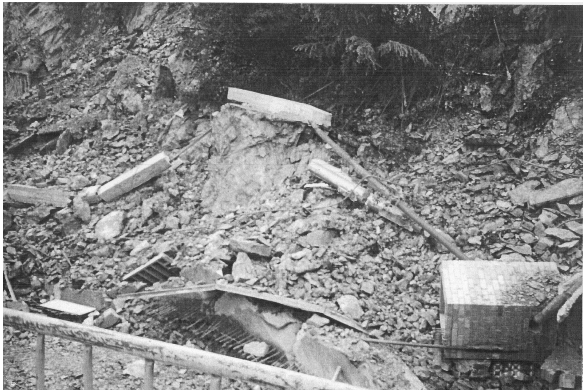
Figure 8. Detail of the failed wall. Parts of the broken piles and cap beam can be seen scattered on the ground surface.
