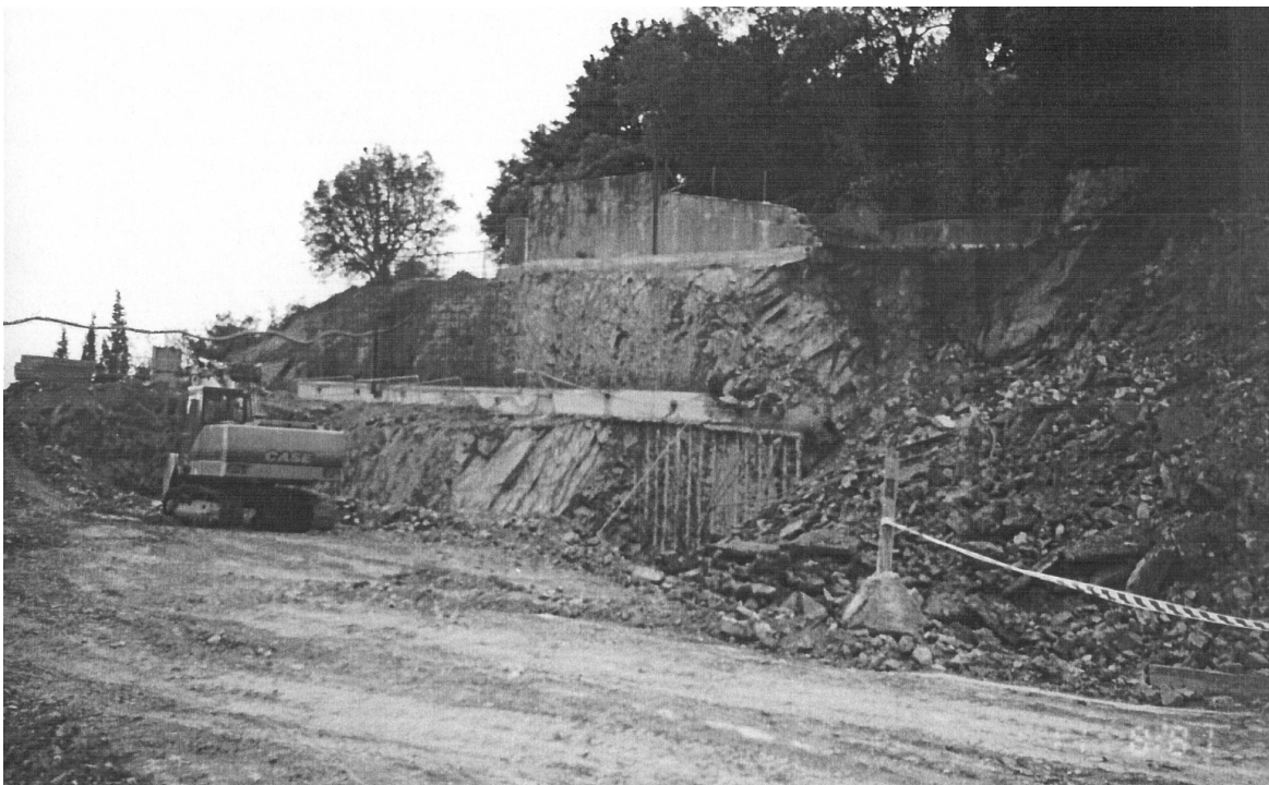
Figure 7. View of the collapsed wall. The intact part of the wall with the cap beam can be seen on the left, and the failed part on the right.
