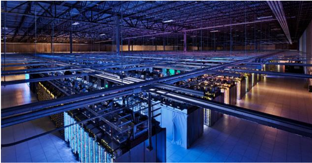
Fig. 4 An overhead view of rows of servers inside the Google data centre in Council Bluffs.
