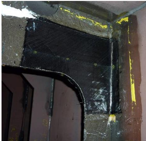
Figure 1.1: Example of a carbon fibre patch applied to a defected steel transverse frame.
