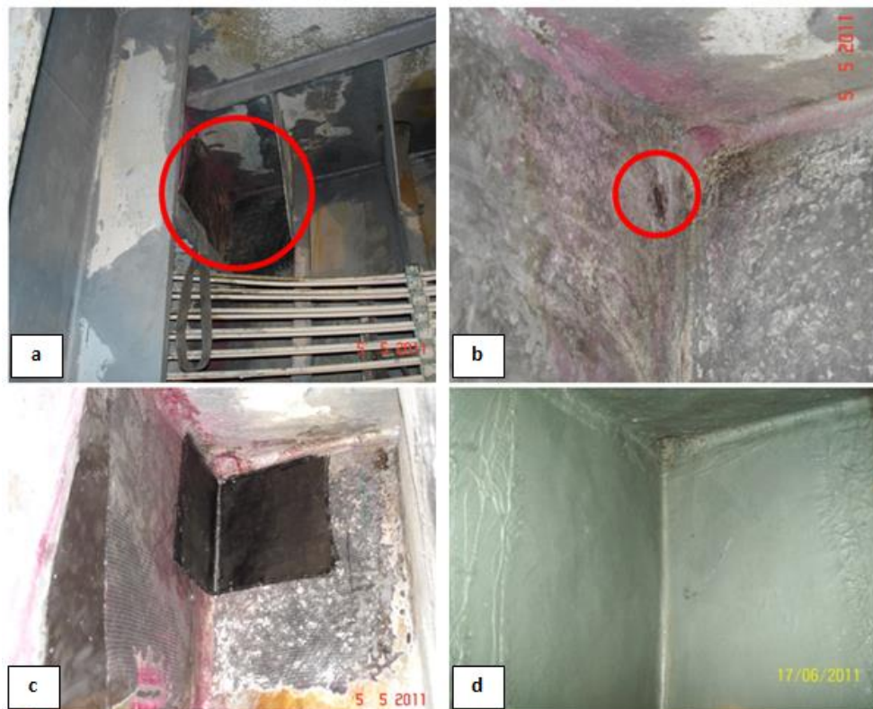
Figure 1.14: Area of damage (pictures a and b), lamination of the repair (c), finished coated repair (d).
