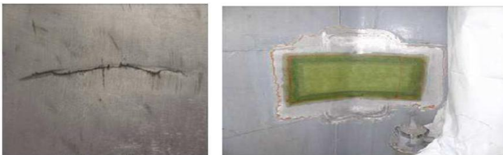
Figure 1.13: Crack in aluminium superstructure and carbon / epoxy patch.
