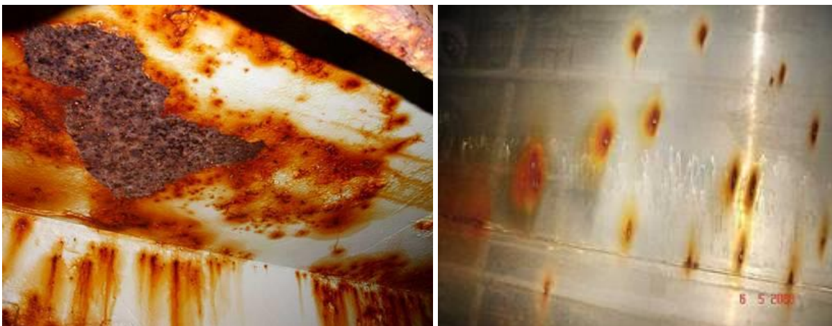
Figure 1.19: General corrosion due to coating failure (left) and pitting corrosion (right).
