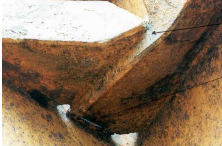
Figure 1.18: Arrows pointing to fatigue cracks at bracket.
