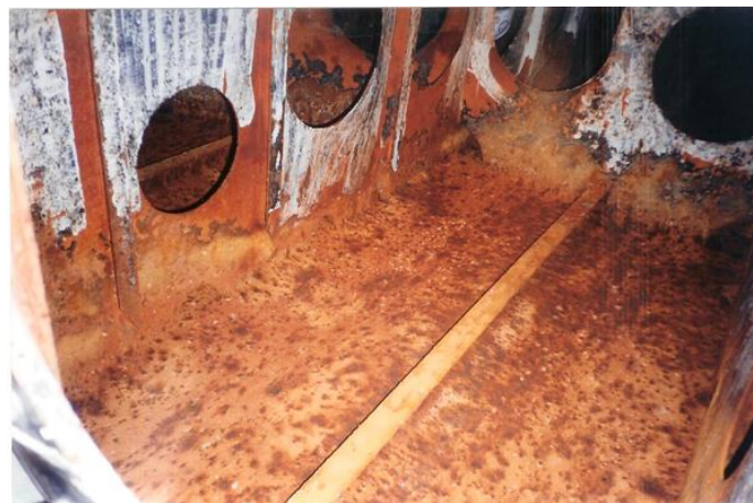
Figure 1.17: Defects in water ballast tank.
