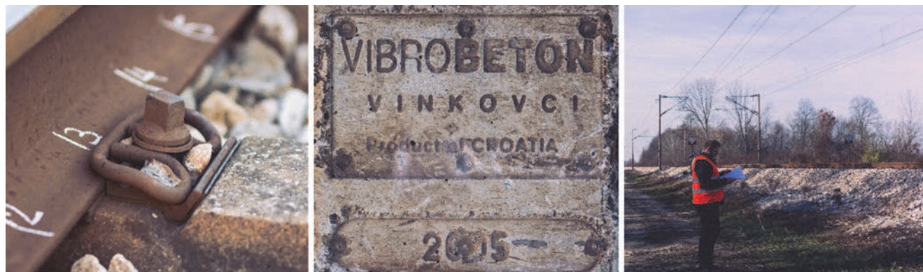
Figure 9. Rail fastened with elastic clip SKL-8 (left side), reinforced concrete sleepers at test section (centre) and ballast prism (right side)
