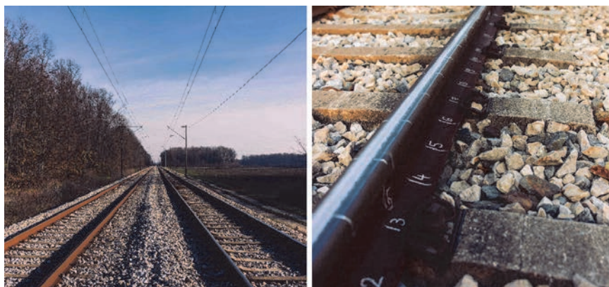
Figure 8. Double track rail line Vrpolje – Ivankovo (position: KM 183+900) (left), and the rail installed at the same section (right)
