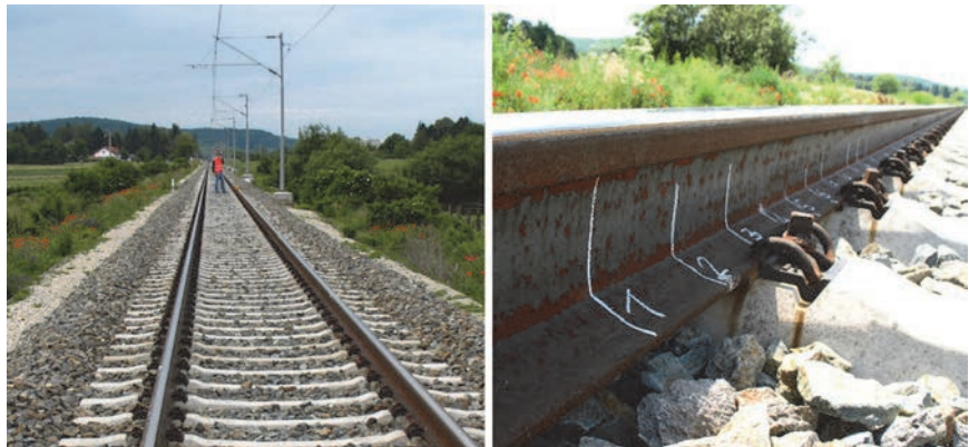
Figure 10. Koprivnica – Križevci single track railway line (left) and installed rail 60E1 (right)
