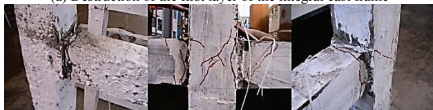
(b) Destruction of the second layer of the integral cast frame
