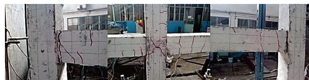
(a) Destruction of the first layer of the strut story-adding framework
