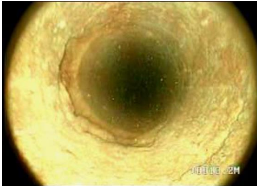
Figure 1: Shear offset imaged in large diameter borehole.
